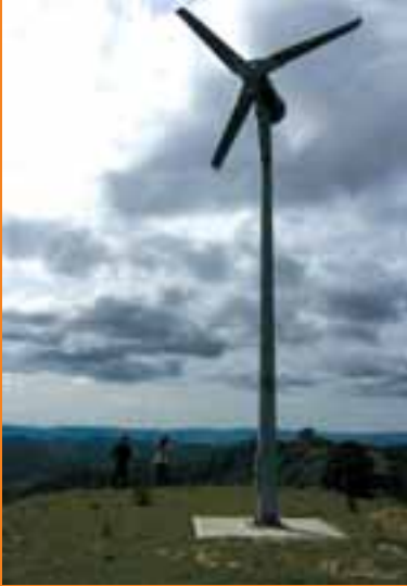
The Proven 2kW wind turbine installed on a hill at Totara Valley. Power generated by the wind turbine will be used to produce hydrogen which will be delivered via a pipeline to a fuel cell at one of the farms.
