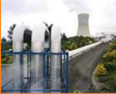
Cooling Towers, Ohaaki Geothermal Power Plant
