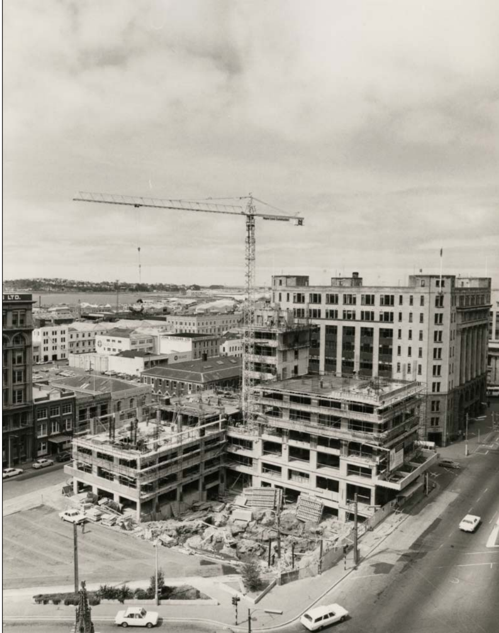
No. 827. John Wickliffe House, photographs of building during construction, 261-271 Princes Street, Dunedin, I.G. Dunn architect, Dalziel Architects records, 1974-1976, MS-2931/090, Archives & Manuscripts Collection, s14-543b.
