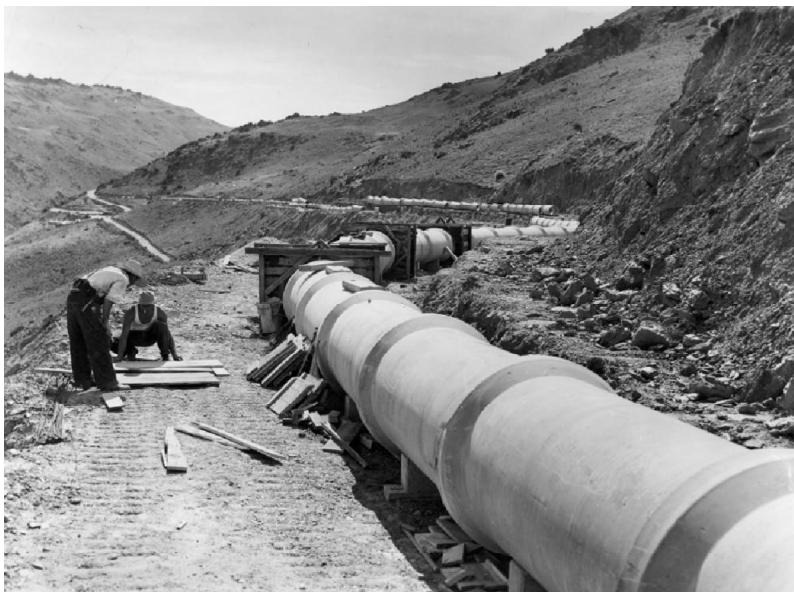
Earlier power schemes were noted for 'small stations and long pipelines'. Here, Ministry of Works men construct the pipeline to the Fraser River Scheme, near Clyde, in the 1950s. [Photo J.F.Shepherd & ODT]
